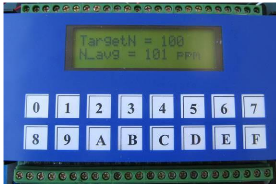
Figure 12. Controller displaying the target nitrogen concentration and the average measured concentration during fertilizer injection.
