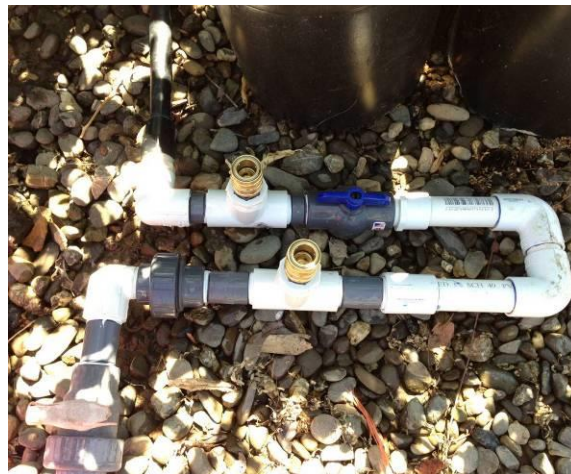
Figure 9. Quick connect adapters allow a mobile injector to be connected and disconnected from a hydrozone.
