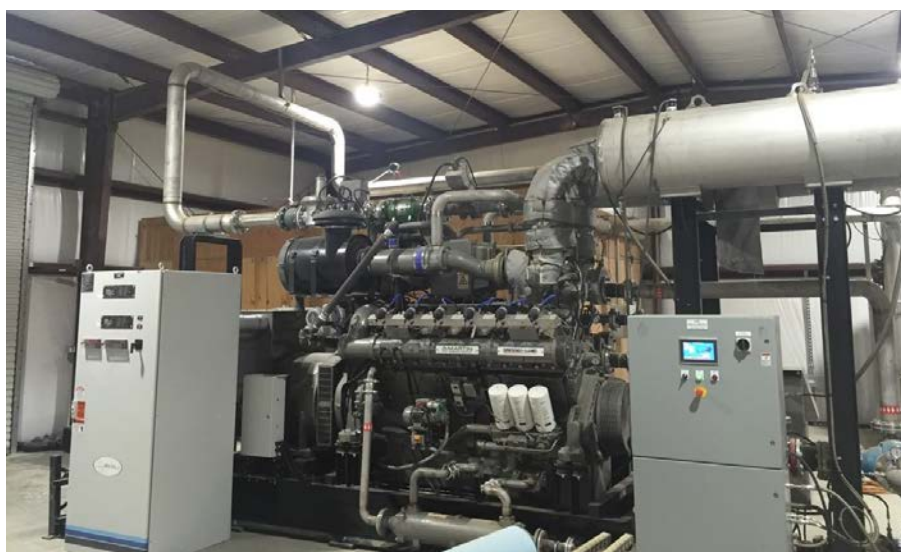
Image 6. Installed electrical genset at Verwey-Madera Dairy.
