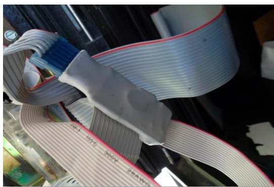
Photo 14: Skimming device installed inside a fuel dispenser cabinet
