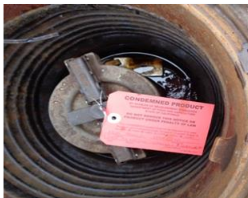
Photo 22: Underground storage tank sealed with a red tag to prevent new deliveries or removal of condemned product
